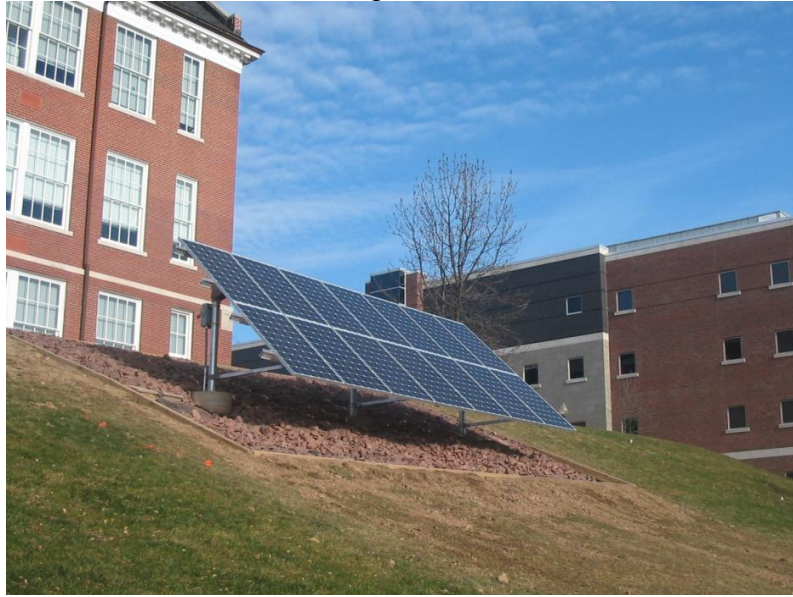
Figure 1: Newly installed 14-panel solar array, with Ben Franklin Hall and Hartline Science Center in the background (left and right, respectively).
